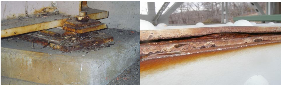
Corrosion Frozen Crevice Corroded Bearing
