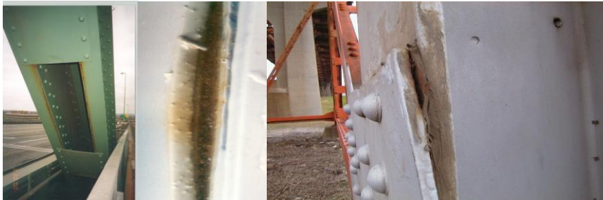
SSPC SP 10, 3 coat Organic ZEU System (left) Inorganic (Right) after 1 year
