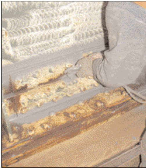
Pack rust can rapidly develop and cause considerable forces to be exerted against adjacent steel members.
