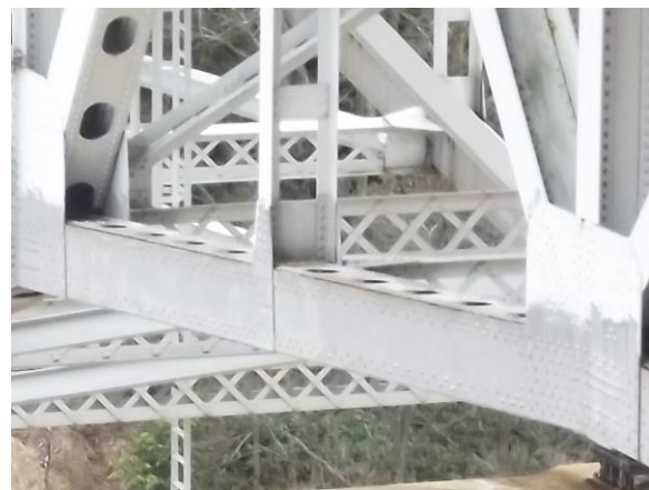
After 10 years – no active crevice corrosion
