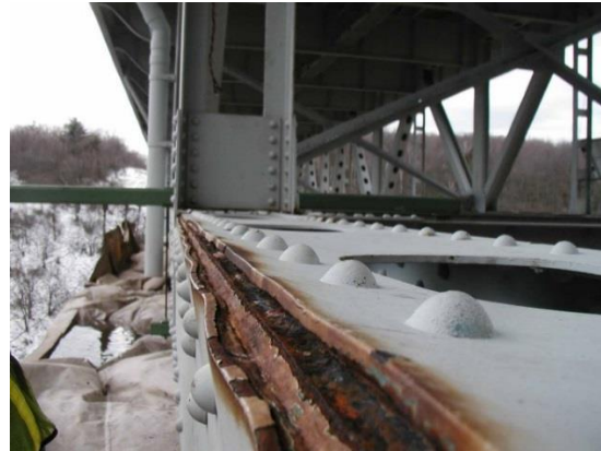
3” Pack rust bent steel plates and overstressed rivets – in all lower chord members
