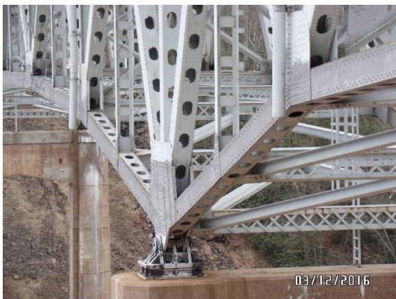
After 10 years – no active crevice corrosion
