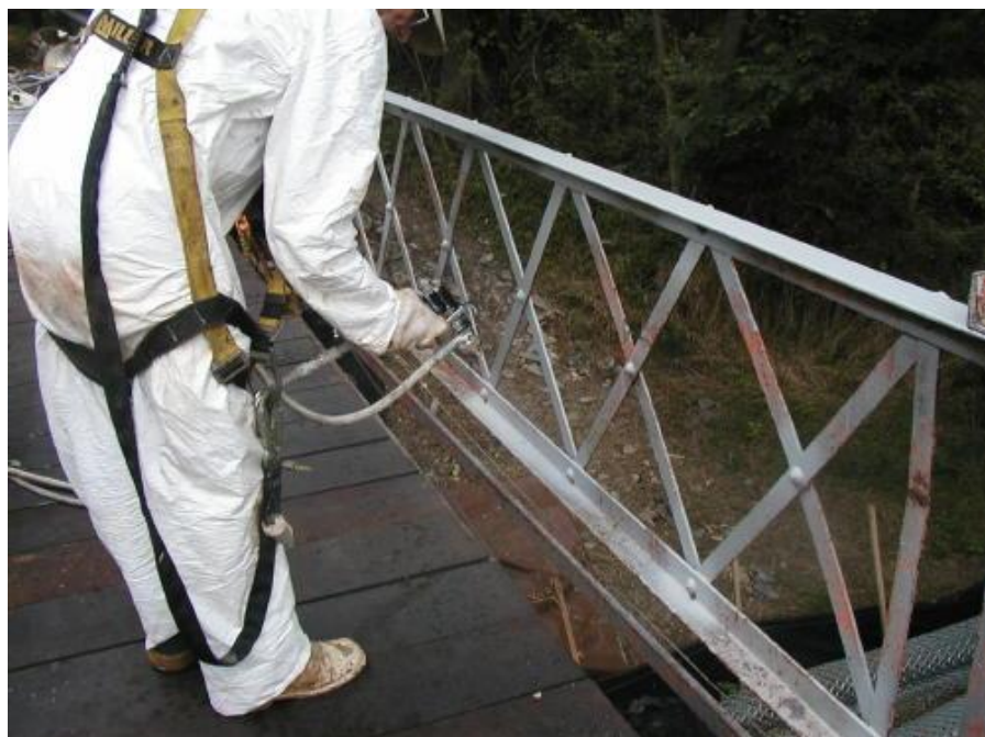
Photo 16 – Applying TR2100 Topcoat, for caulk/stripe coat and spot priming over bare steel and tight rust.
