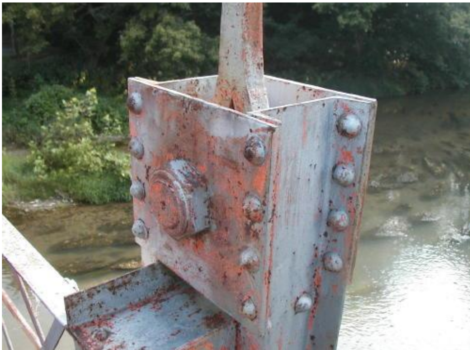
Photo 10 – Bottom of tie rod assembly cleaned and ready for painting. (see Photo 25)
