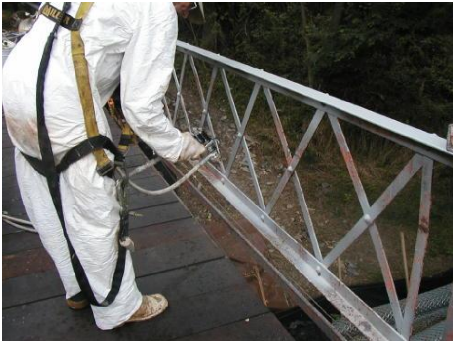
Photo 16 Applying TR2100 Primer/Topcoat, for caulk/stripe coat and spot priming over bare steel and tight rust.
