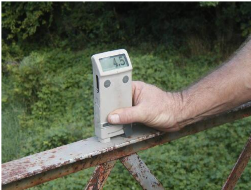
Photo 14 Film thickness gage shows 4.5 mils of existing tightly adhered lead-based paint.
