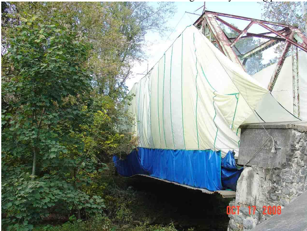
Photo 6 – Containment for pressure wash cleaning and collection of lead paint containing chips of paint and corrosion debris
