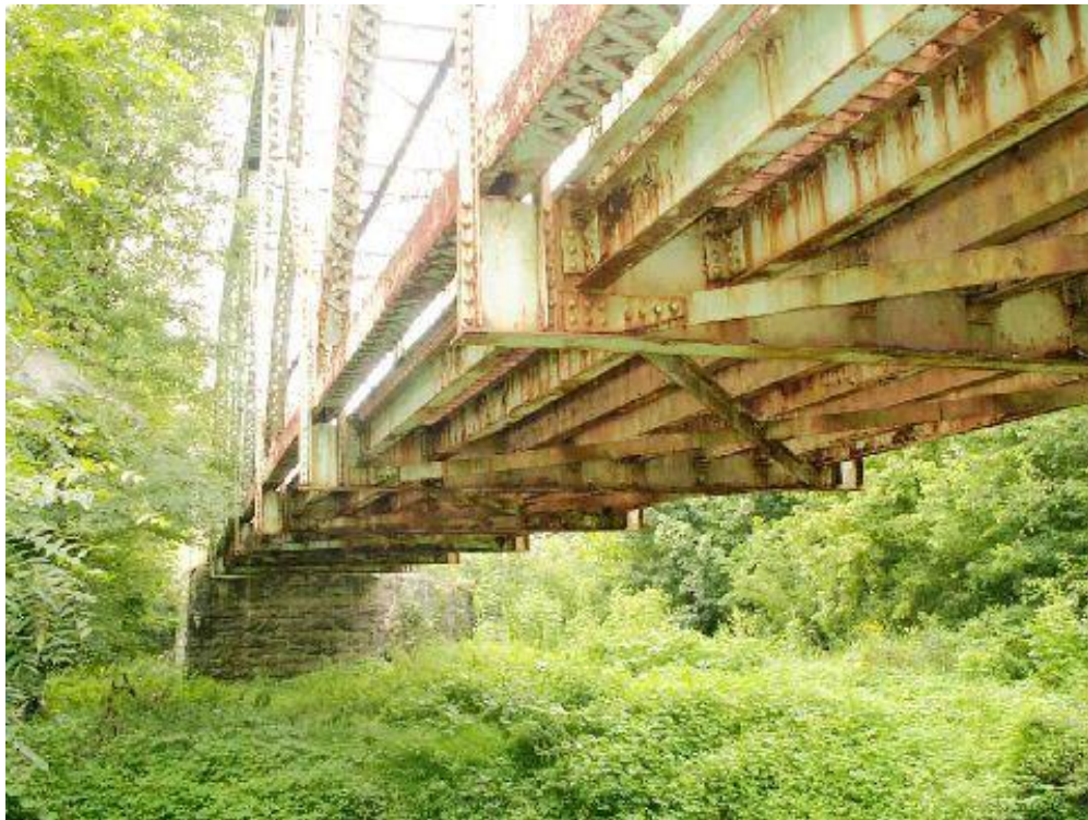
Photo 4 – The underside of one span of the truss, before cleaning and coating with Termarust.
