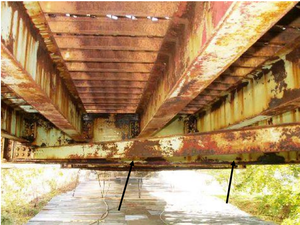
Photo 10 – After pressure washing – some scale rust remains on some members under the deck, which must be mechanically removed, because there is active corrosion under it.
