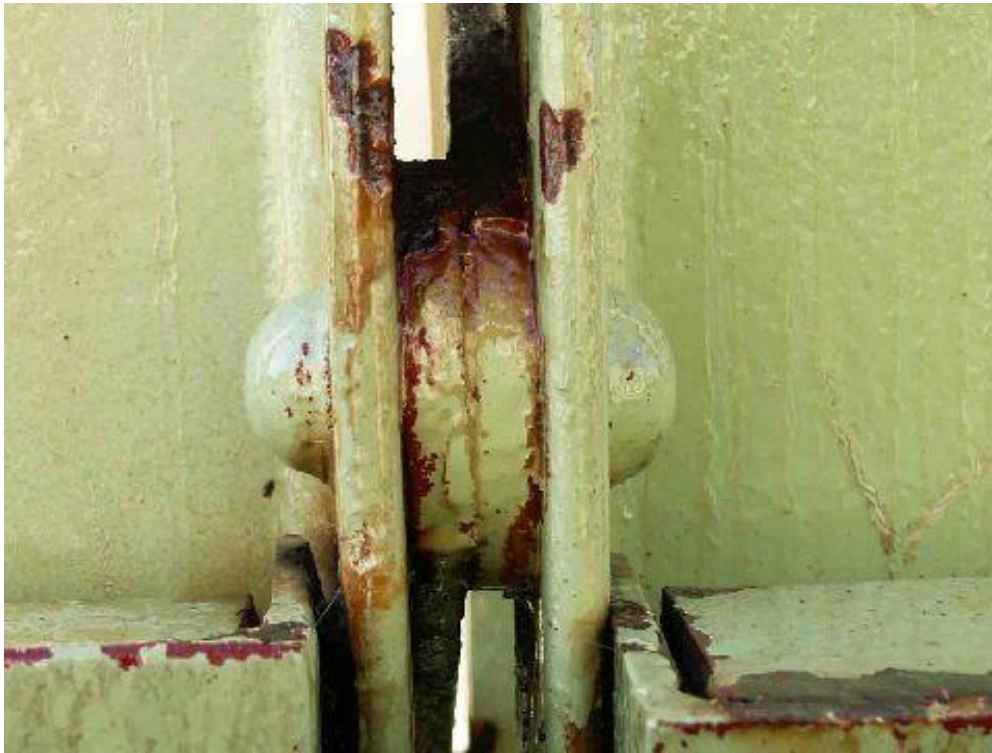
Photo 7 – After pressure washing – loose paint and loose corrosion debris has been removed.
