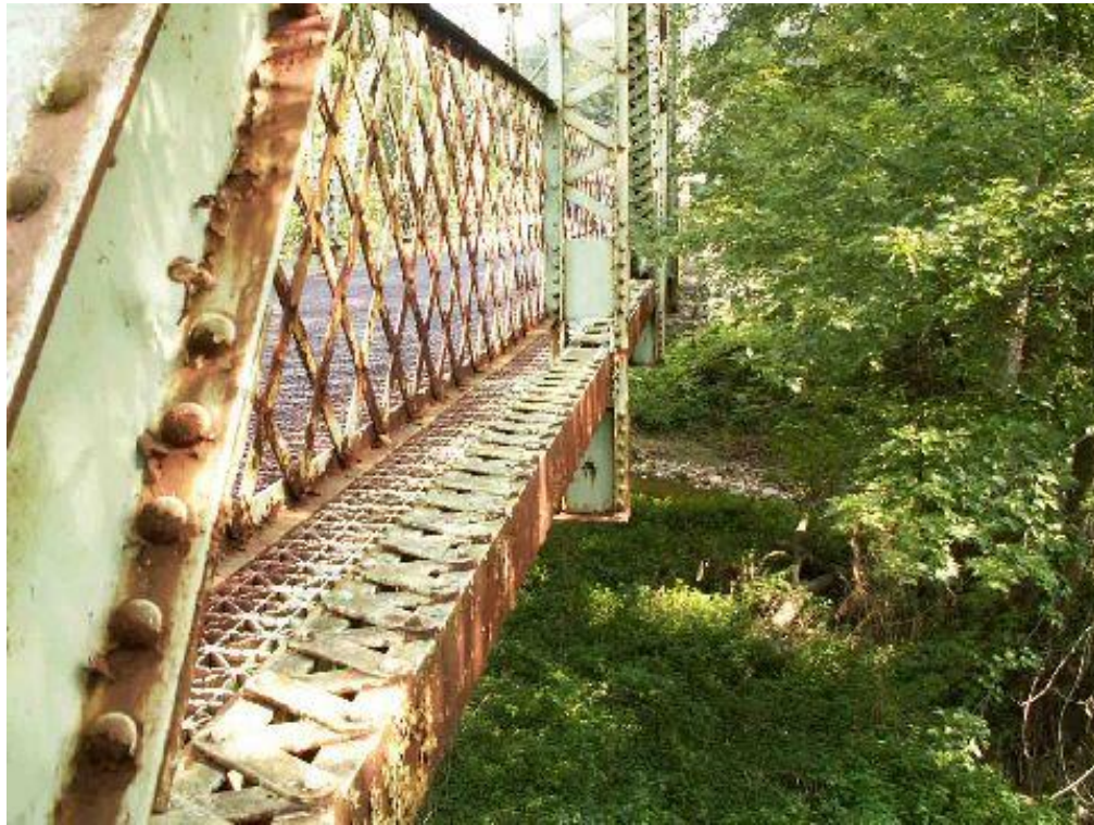
Photo 3 – View of outside of the truss, before cleaning and coating with Termarust
