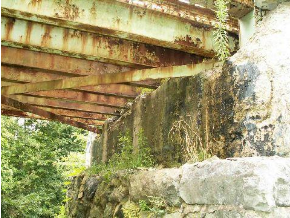
Photo 5 – Underside of the deck, at the pier. The ends of four of the longitudinal beams had corrosion-caused holes in the webs. The webs were strengthened by welding plates to both sides.
