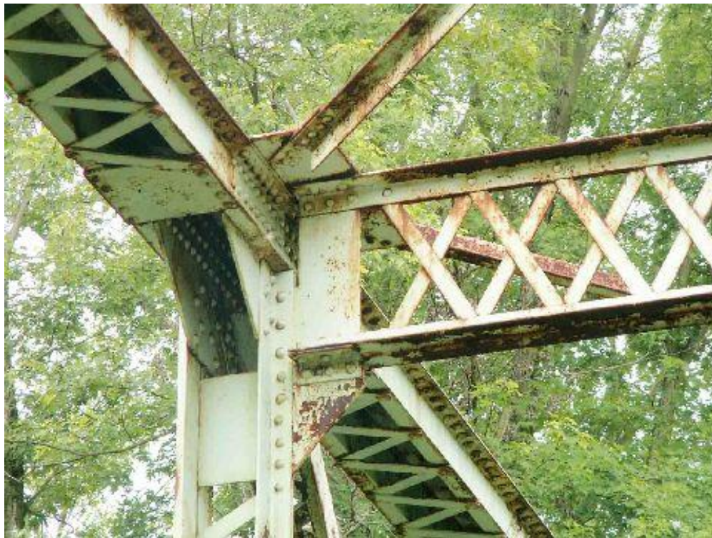
Photo 2 – Upper portion of the truss – showing corrosion and some pack rust.
