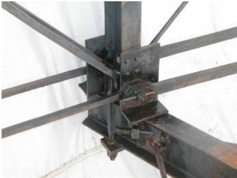
Photo 14 TR2200 Penetrant has been applied to the connection, before application of the TR2100 Topcoat.
