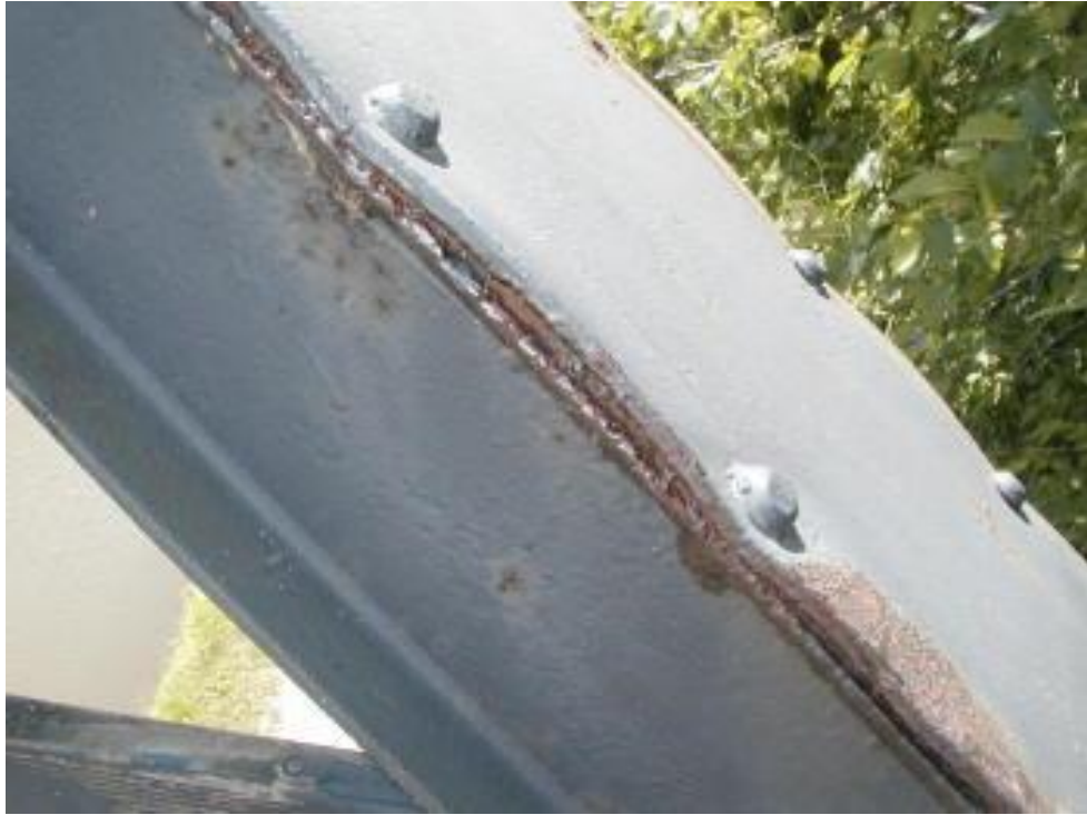
Photo 5 Close-up of pack rust that has bent the cover plate.
