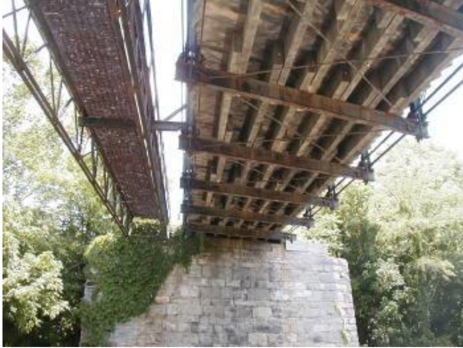
Photo 3 Underside of the bridge showing transverse floor beams and longitudinal timber beams
