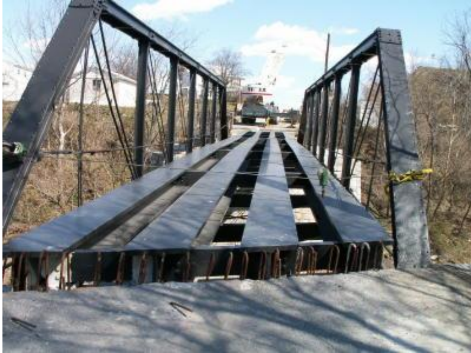
Photo 17 The truss has been painted and the new longitudinal beams have been installed.
