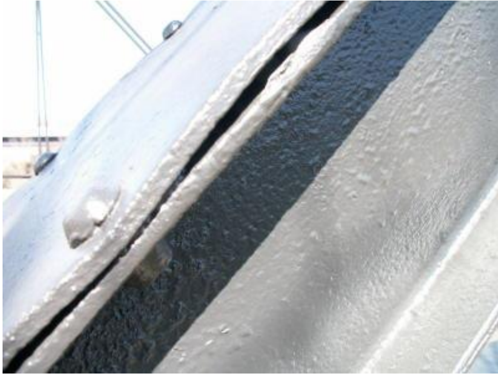
Photo 19 Close-up of connection with most of the pack rust removed before painting.
