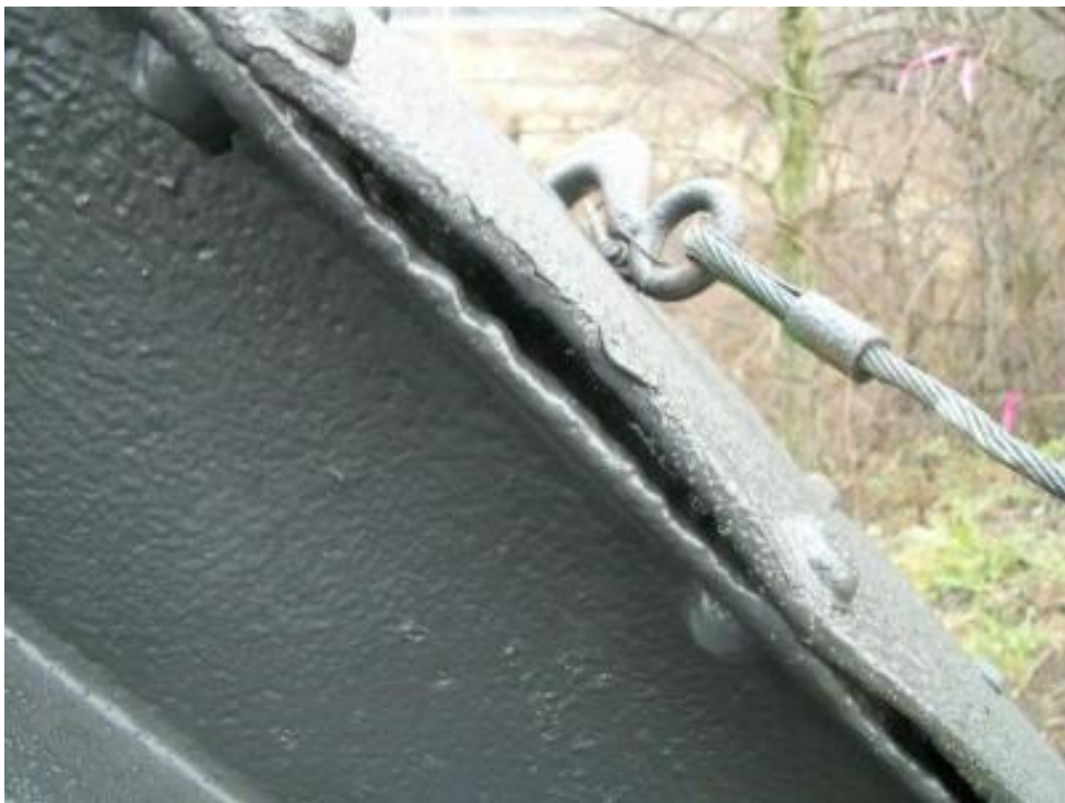
Photo 20 Close-up of connection with most of the pack rust removed before painting.
