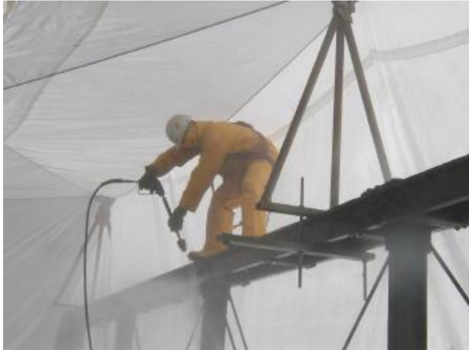
Photo 10 5,000 psi pressure washing of the truss, with Chlor*Rid in the final rinse water.
