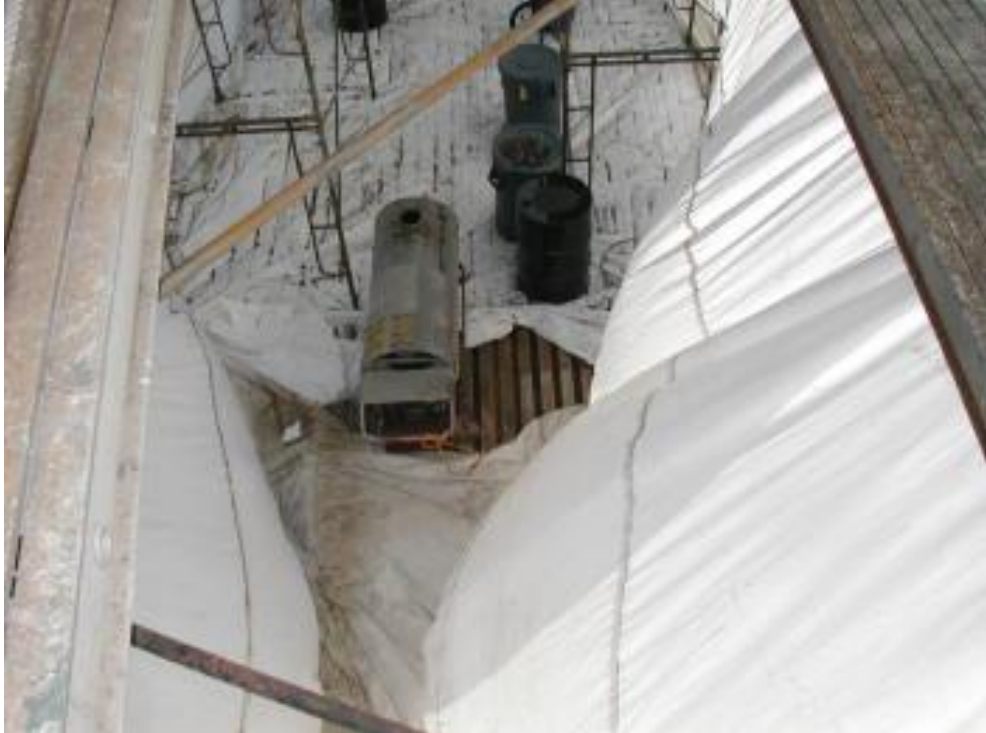
Photo 11 A large heater was used to maintain a minimum 50°F steel temperature for painting.
