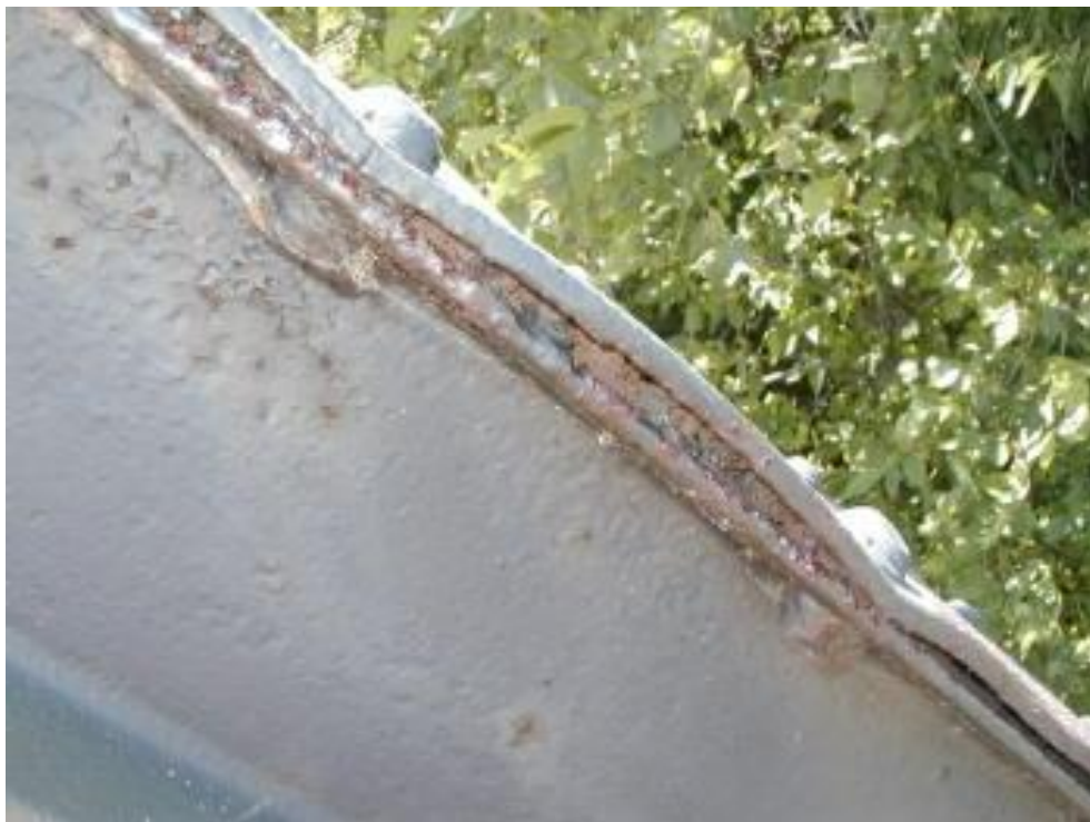
Photo 6 Closer view of the pack rusted connections.
