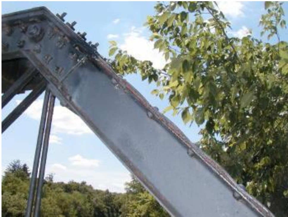
Photo 4 Edge of front truss member with crevice corrosion and pack rust that has bent the cover plate and stressed the rivets.
