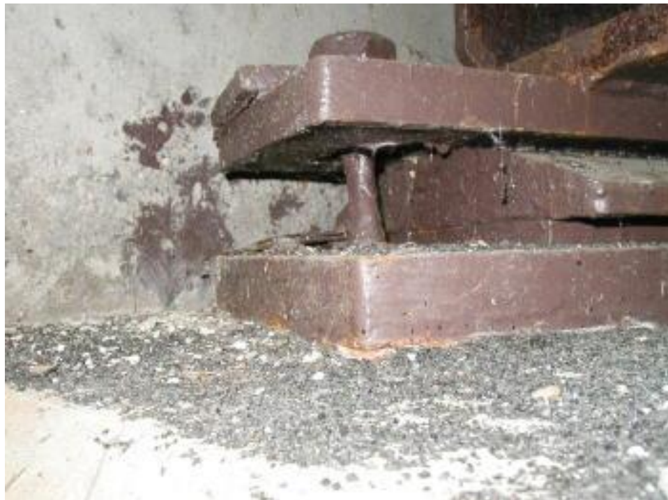
Photo 14 Condition in May 2005, no corrosion of the bearings or anchor bolts.
