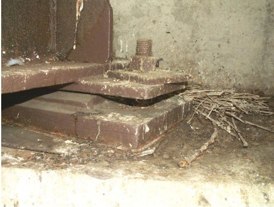
Photo 17 Condition of an exterior bearing in September 2007, after 6 years (No corrosion or rust staining)
