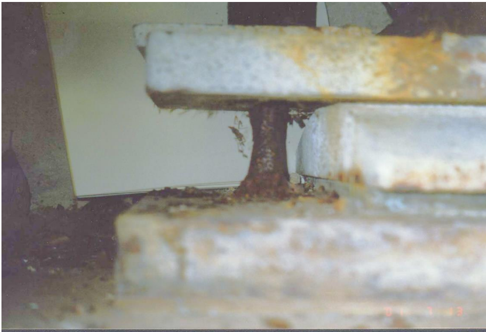
Photo 6 Corrosion ring/shell around anchor bolt has fallen off revealing substantial loss of cross sectional area of the bolt. ( Compare with Photos 11, 14 and 21 )
