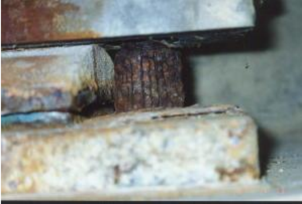
Photo 5 Existing condition of anchor bolts severe corrosion Corrosion ring/shell has expanded and cracked vertically but it has not yet fallen off (as seen in the next photo)
