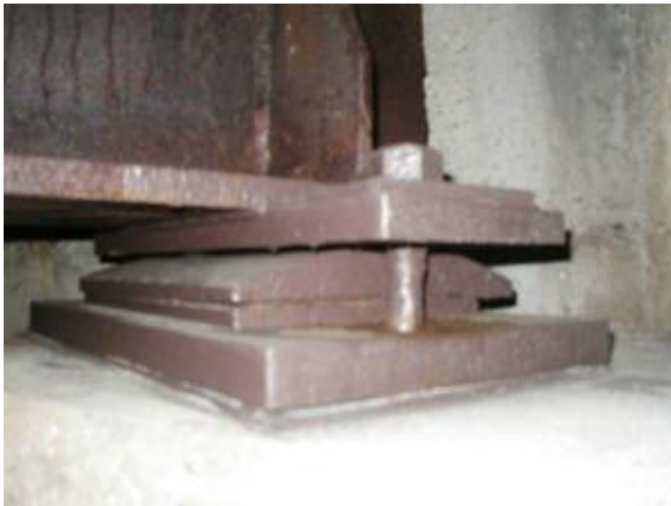
Photo 12 Condition in November 2003, no corrosion after 27 months.
