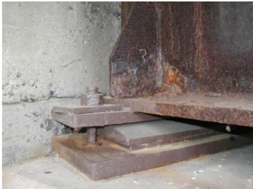
Photo 16 Condition in May 2005, no corrosion of the bearings or anchor bolts. (Rust staining is from the underside of the top bearing plate and inside of holes in plates)
