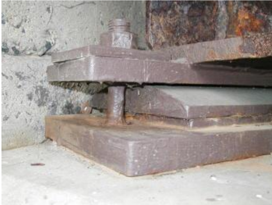
Photo 15 Condition in May 2005, no corrosion of the bearings or anchor bolts. (Rust staining is from inside of hole in upper bearing plate)
