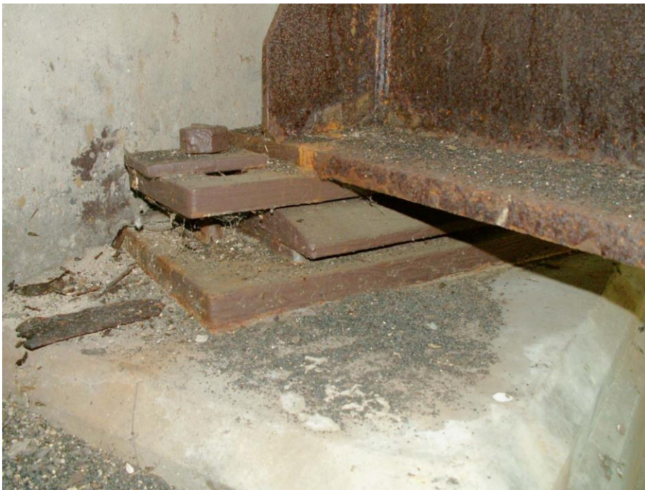
Photo 20 Condition in September 2007 after 6 years (Rust staining is from the underside of the top bearing plate and inside of the holes and rusting of the unpainted A-588 steel beam)
