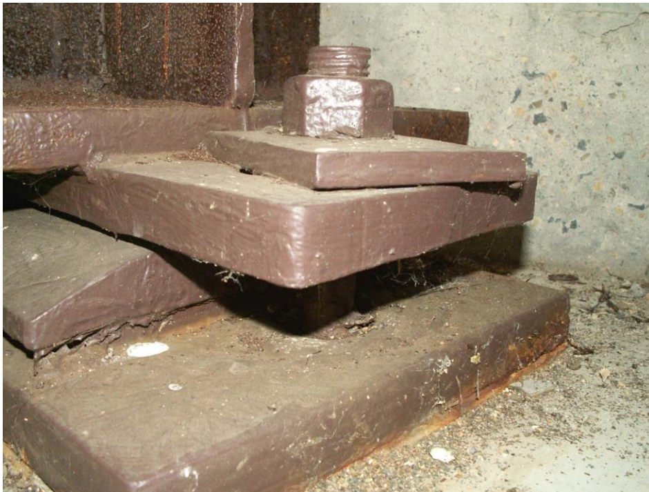
Photo 18 Condition in September 2007 after 6 years (Rust staining is from the underside of the top bearing plate, inside of holes in plates and under base plate)
