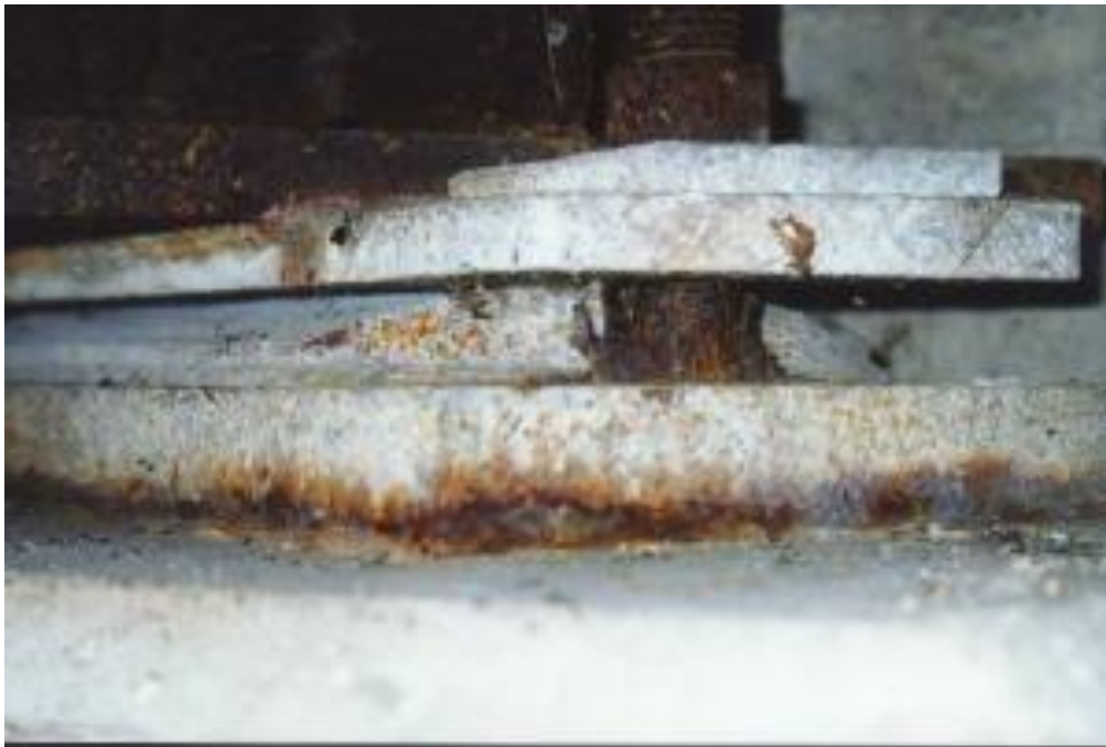
Photo 4 Existing condition of anchor bolt, note corrosion.
