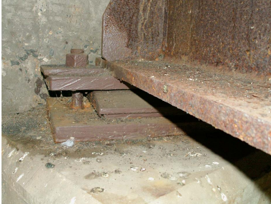
Photo 21 Condition in September 2007 after 6 years (Rust staining is from under underside of plates and inside of holes and the A-588 beam ( Compare to Photos 6, 11 and 14 ))
