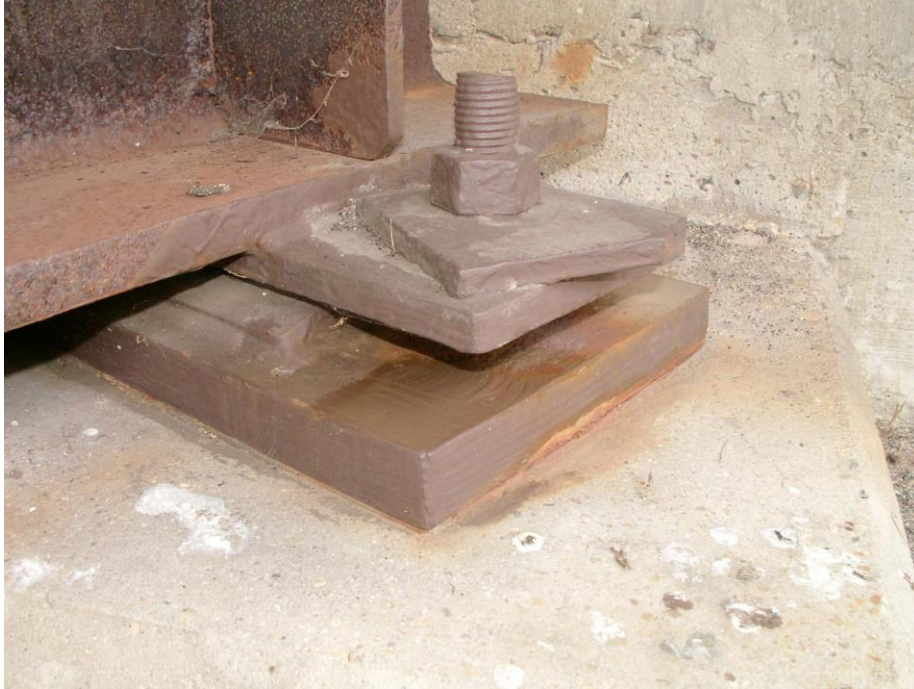
Photo 19 Condition in September 2007 after 6 years (Note that rust staining on top of the front corner of the base plate has been washed off paint under it is in excellent condition)
