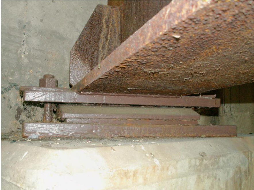
Photo 22 Condition in September 2007 after 6 years (Rust staining is from unpainted A-588 steel beam)
